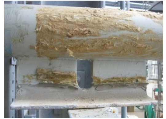
Welded Pipe Support
